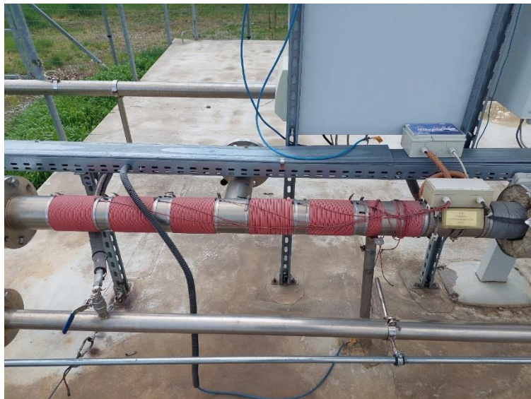
Figure 4. Electromagnetic system protecting the stainless-steel pipeline section leading to the degasifier (Nagyszénás)
