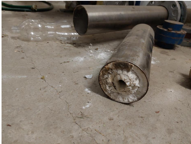
Figure 3. Scaling in the geothermal system (Nagyszénás)
