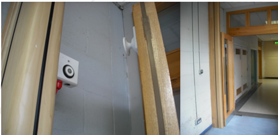
9.9. Example of electromagnetic hold-open device used to hold fire doors in corridor open while in normal use. Activation of the fire alarm or a power cut deactivates the electromagnetic hold-open device and the doors close under the action of standard door closers
