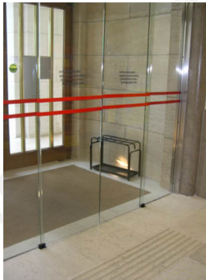
8.4. Visual marking the glazed door prevents accidents
