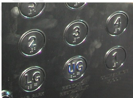
8.5. Tactile control panel in the elevator
