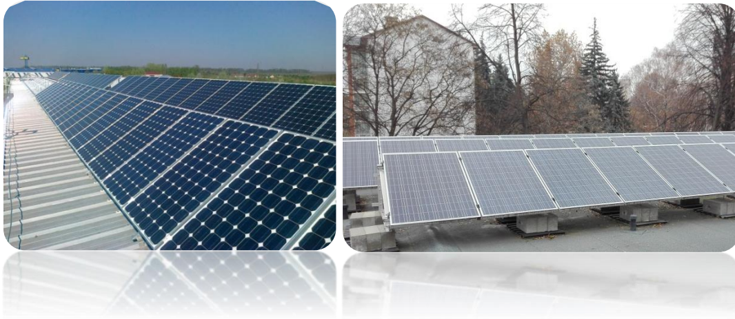
1. foto Installed monocrystalline and polycrystalline PV cells in No.2 and No.4 system
