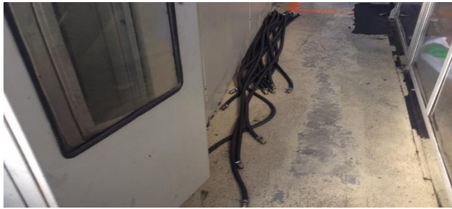
Figure 35.: Misplaced Cables and Wires [110]
