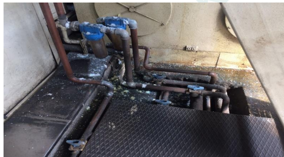
Figure 33.: Improper maintenance of pipes and valves [110]
