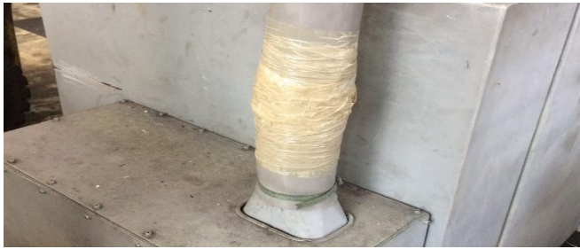
Figure 37.: Improperly maintained pipe [110]
