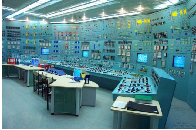
Fig. 2.1 The real control room (source: [114])
