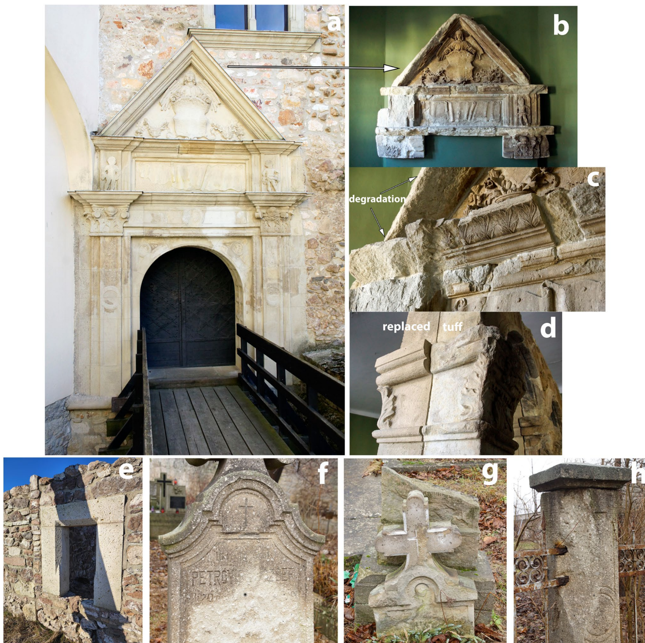
Fig. 7 Degradation of decorative stones. Vágáshuta Tuff : (a) Large gate of Red Tower (Sárospatak Castle) replaced by artificial material. (b-c) Original degraded stones of the gate in the museum. (d) Unique combination of original and artificial stone showing the difference in
