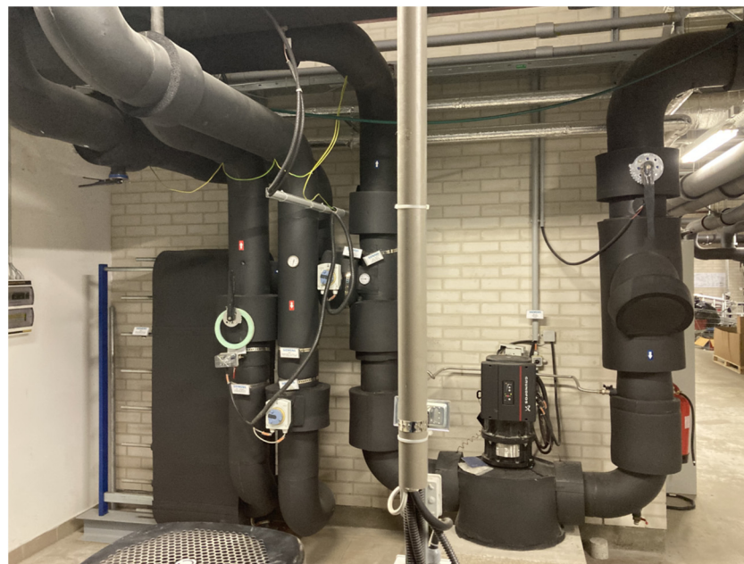
Figure A7. Heat exchanger.
