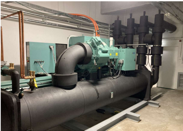
Figure A3. YORK YMC2 type centrifugal compressor water chiller.
