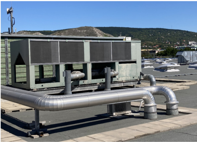
Figure A2. Water chiller.
