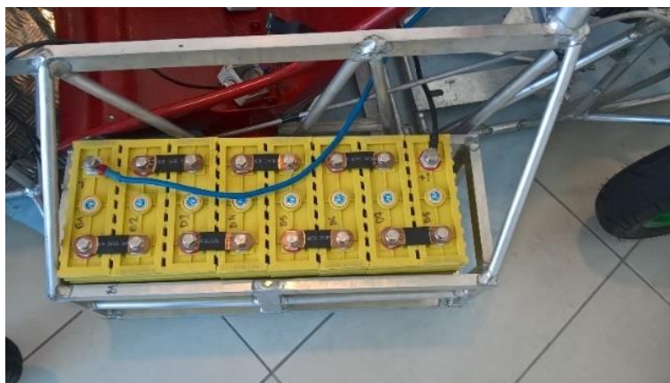
Figure 22.: E-vehicle System of batteries [12]
