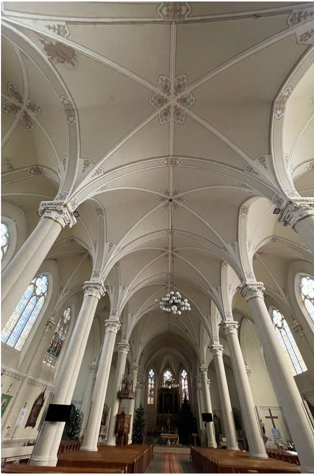
FIGURE 6 Church interior in Bačka Topola. Pillars: Reinforced concrete, transverse arches: Masonry, ribs: Reinforced concrete, panels: Staff (rabitz). Source: Éva Lovra, 2023.
